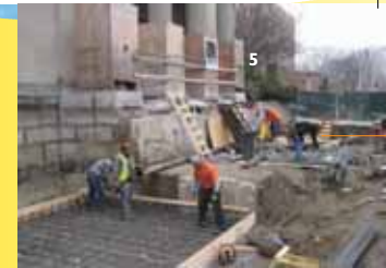
"Steps currently under construction" The restoration of the steps revives the original intent of the Riverway Entrance, which was built in 1925.
